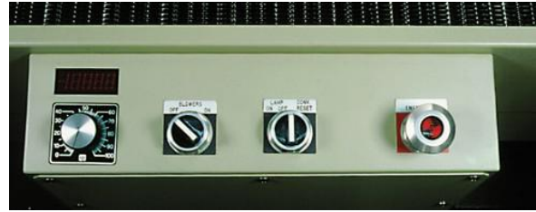
System control panel.
